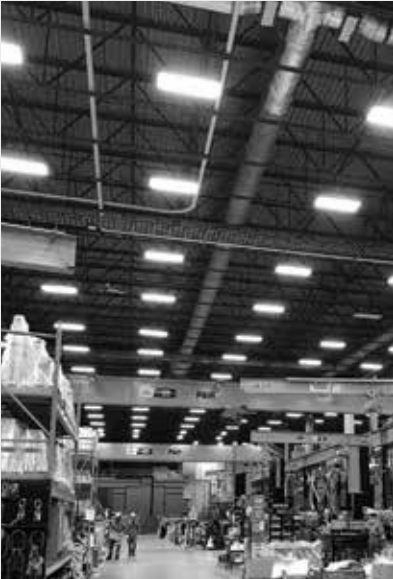
Replacing incandescent light bulbs with LEDs at 15 facilities reduces electricity use and associated GHG emissions.
